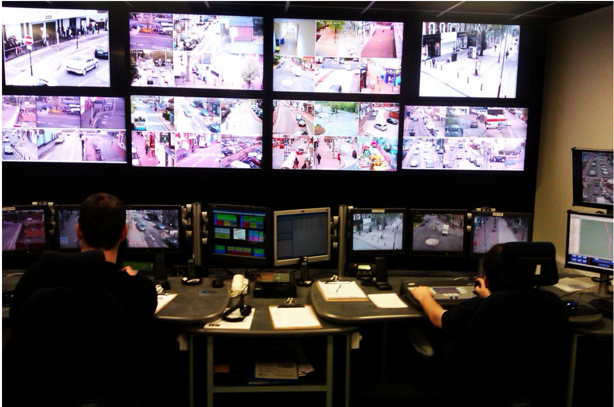
CCTV Control Room
